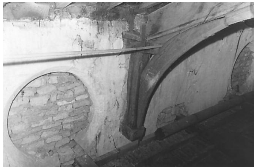
The blocked clerestory windows
