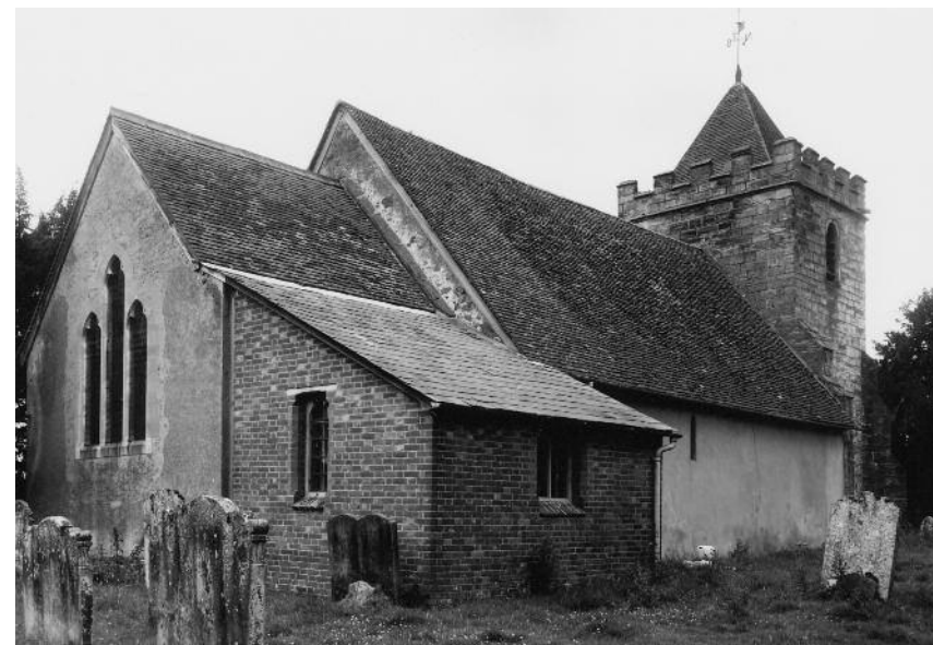
Exterior looking from the north-east, showing the vestry of 1815 and the tiny Norman window in the nave
